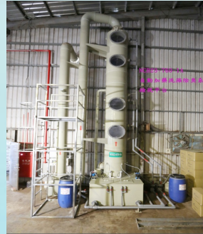
Automatic dosing and deodorization scrubber
